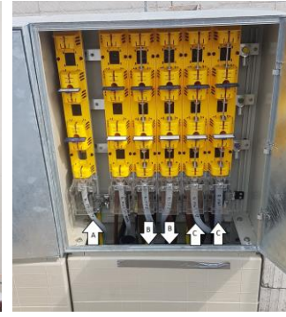
microgrid connection point
