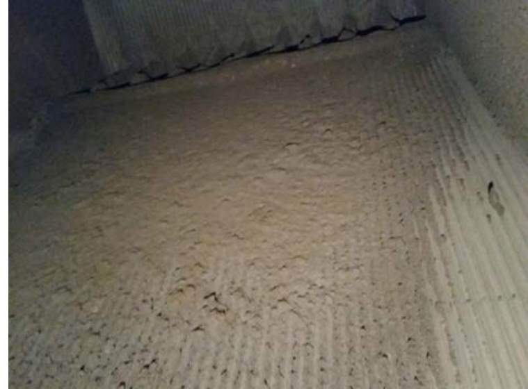
Rear wall of the 2 nd duct against the flow direction after a system operation of 9 weeks
