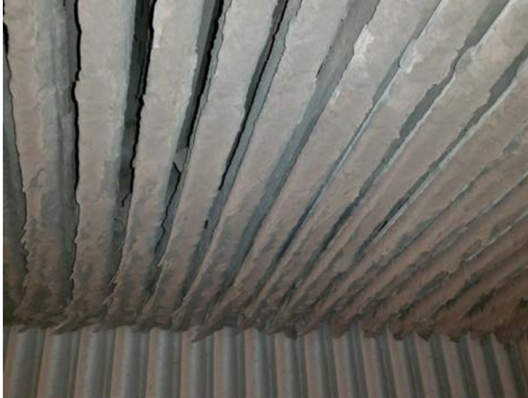
Protective evaporator from below (in the flow direction, luv) after a system operation of 9 weeks
